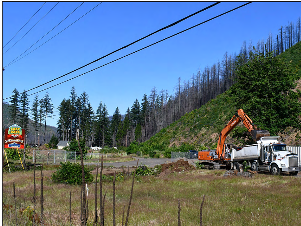
Meili Construction based out of Eugene is the general contractor for the entire Lazy Days rebuild project. Stump removal and grading of the site is now underway, in addition to the community septic work.
