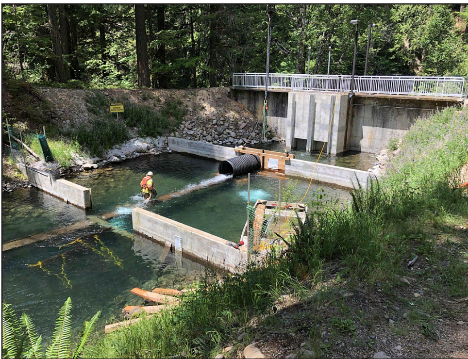
Crews from Wildish Construction built a temporary pipeline/dewatering project at the Carmen Smith Hydroelectric Project as part of a trap and haul project.
