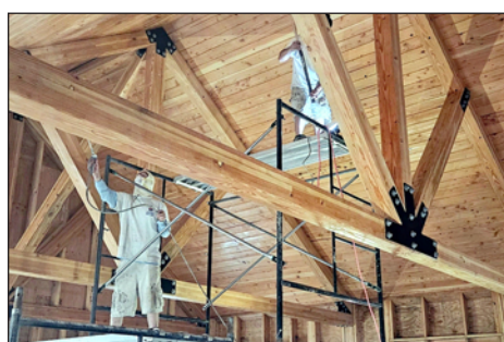
Work continues to progress inside and out at the Vida McKenzie Community Center.
