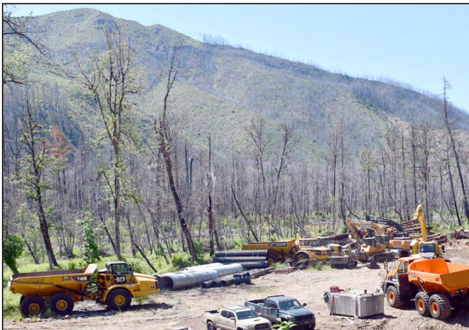
Construction equipment had been gathering as work on the Finn Rock Landing project got underway last Friday.
